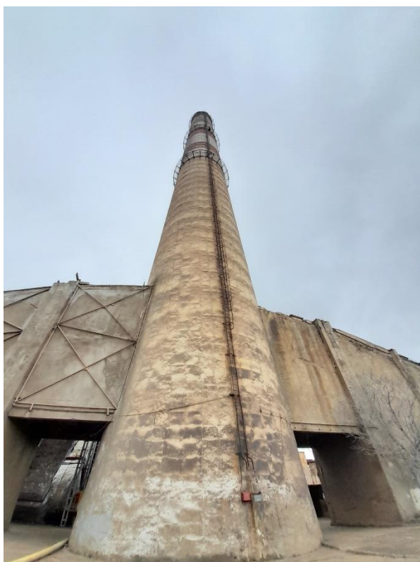
Stack frontside with ladder
