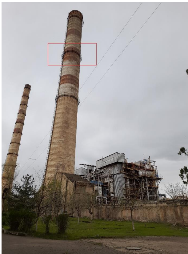
Stack frontside with measuring platform
