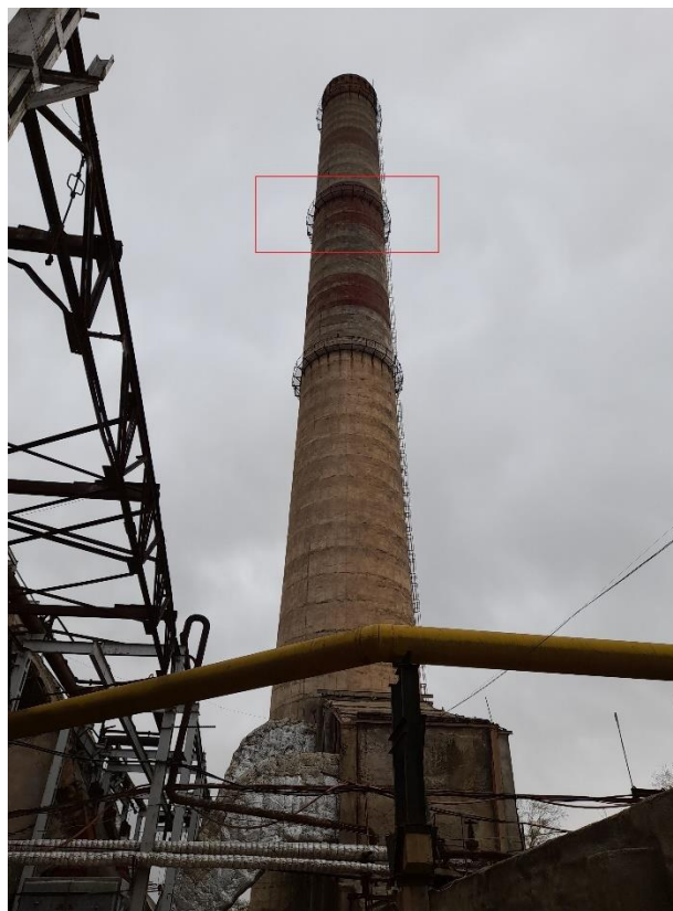
Stack left side with measuring platform
